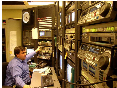
Master Control Room
